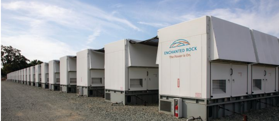
These 123 natural-gas-powered engines enclosed in these modular units provide 50MW of on-demand power.. | PHOTO BY RYAN HALL
